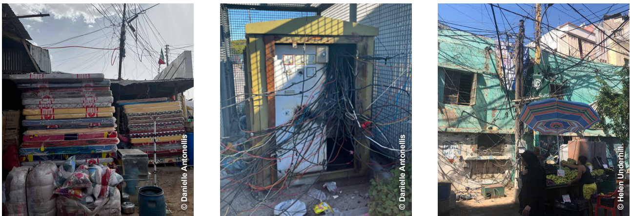
Figure 4: Photographs of unsafe electrical systems in a marketplace in Hargeisa, Somaliland; in an informal settlement in Cape Town, South Africa; self-settled refugee camp in Beirut, Lebanon
