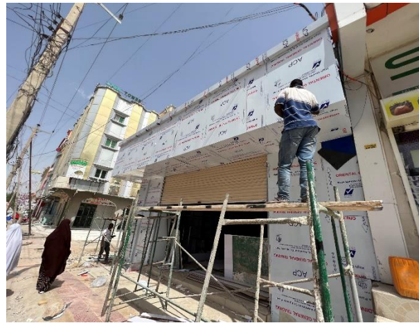
Figure 17: Installation of Aluminium Composite Panels on a building along the perimeter of Waheen market (post-fire image)
